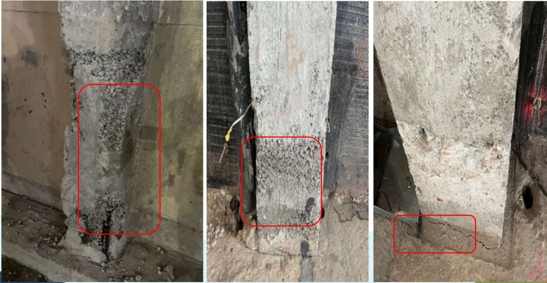
Existing column structures poorly constructed
