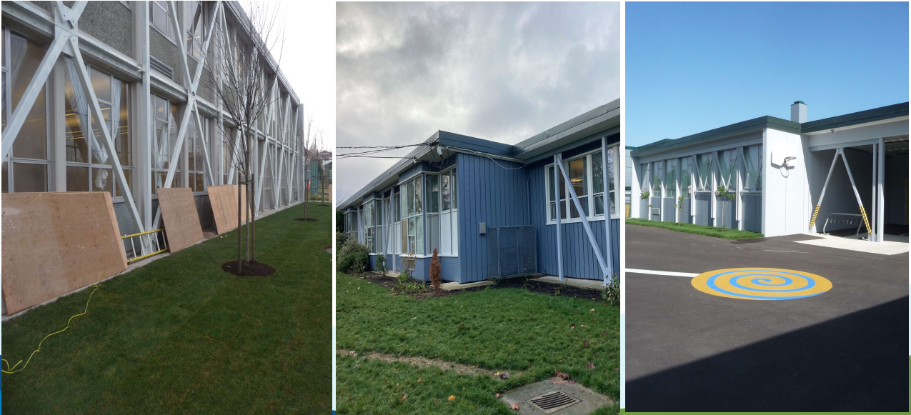
Exterior Seismic Braces
